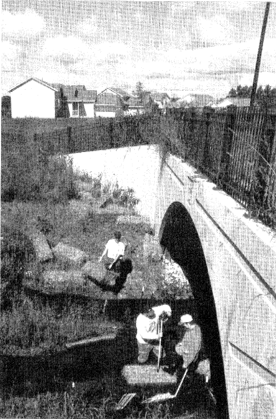
The new Eagle Creek Advisory Committee is assisting with in-stream restoration of the west branch of the creek. Here bales of hay are used to narrow and eventually deepen the creek as it flows under the Independence Avenue bridge.
